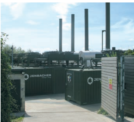
The engines which convert landfill gas into electricity
